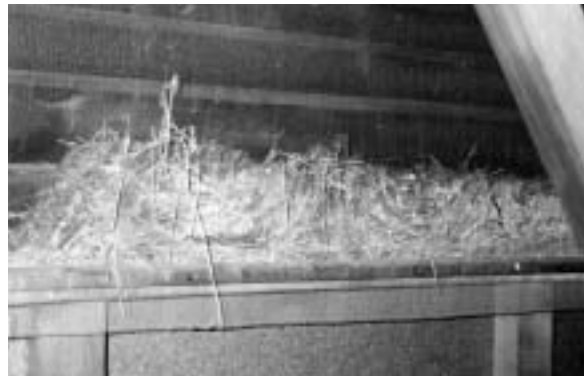
Sparrow nest located in an attic lower vent.
