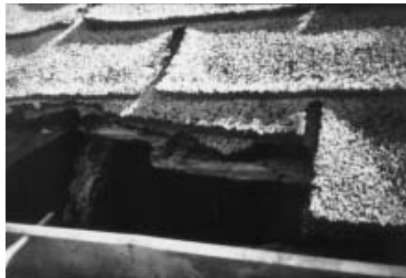
Animal entry point located above fascia board (gutter line) - most likely caused by a raccoon who found soft (rotted) roofing material.
