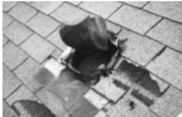
Attic vent destroyed by a raccoon – Notice the hardware cloth installed under vent, which prevented easy access by the raccoon. This is a simple step that can prevent animal intrusion. Better yet, simply install new stainless steel roof vent guards.
